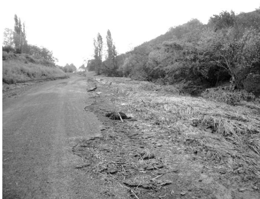
Garden Gulch Road damage, flood 2005
