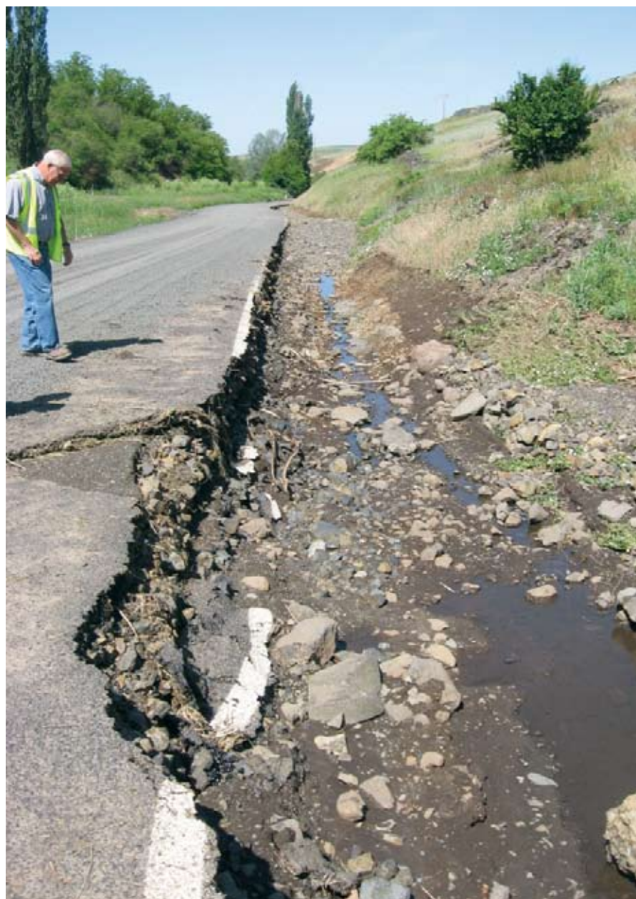
Road Director Doug Moore examines Garden Gulch Road after rainstorm
