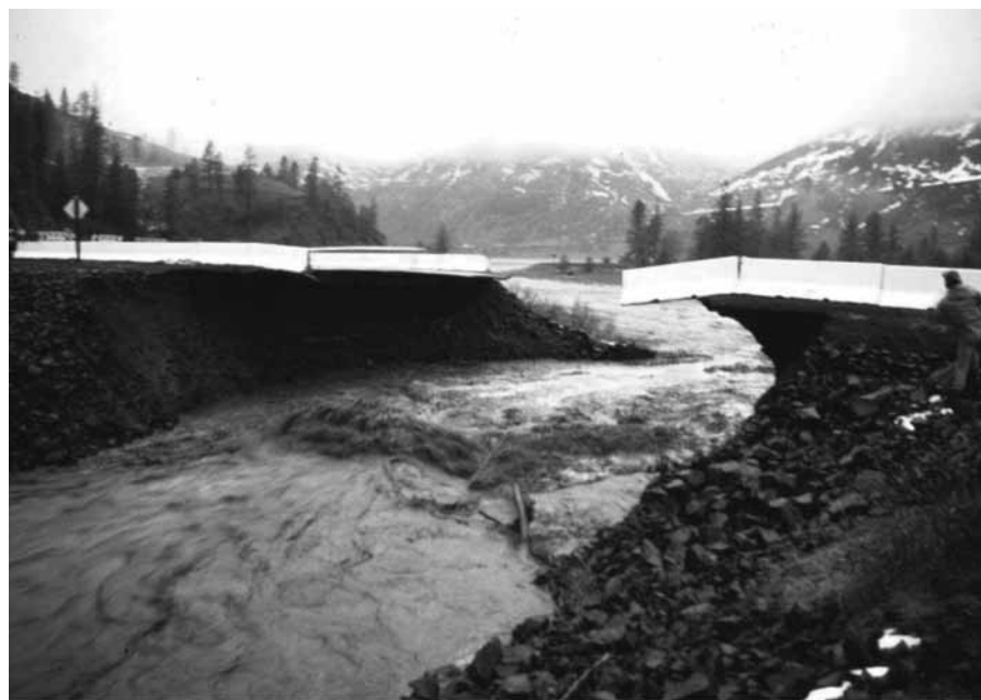
Cottonwood Creek bridge damage, February 1997
