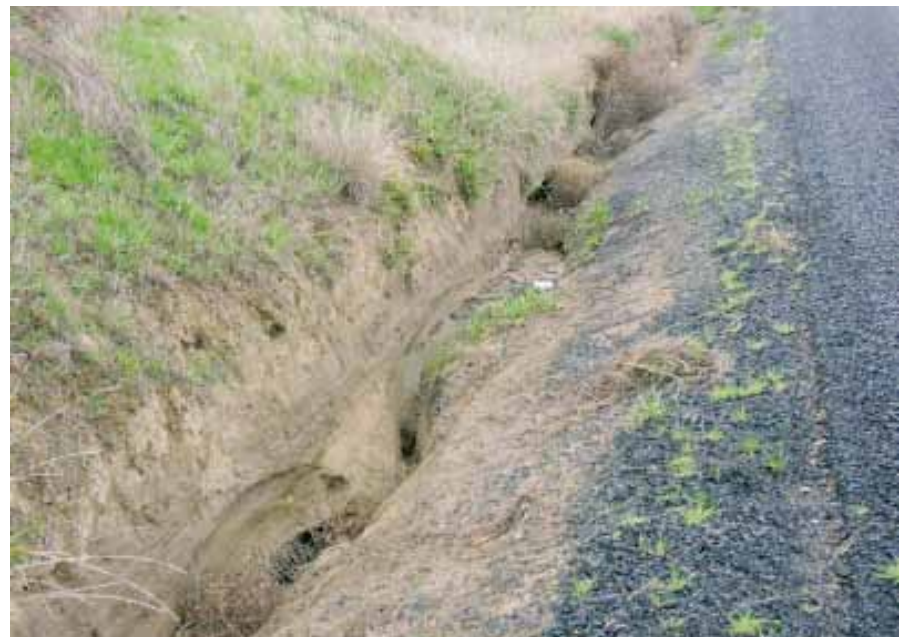
Eroding banks along Vollmer Road
