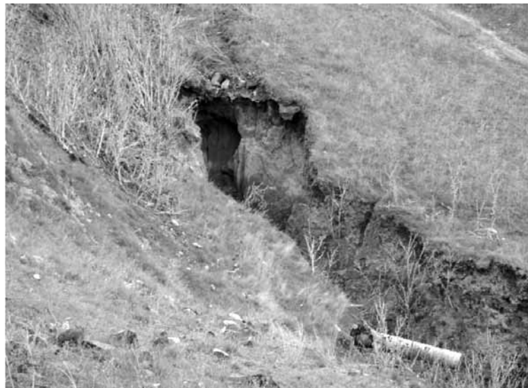
Erosion along Vollmer Road
