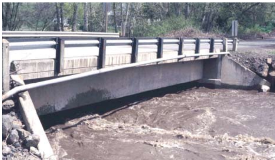
Water levels rise under bridge to Tom Beall Road, Nez Perce County, circa 1996
